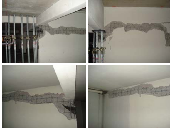
Figure 2. Horizontal failure strip in basement shear walls.
